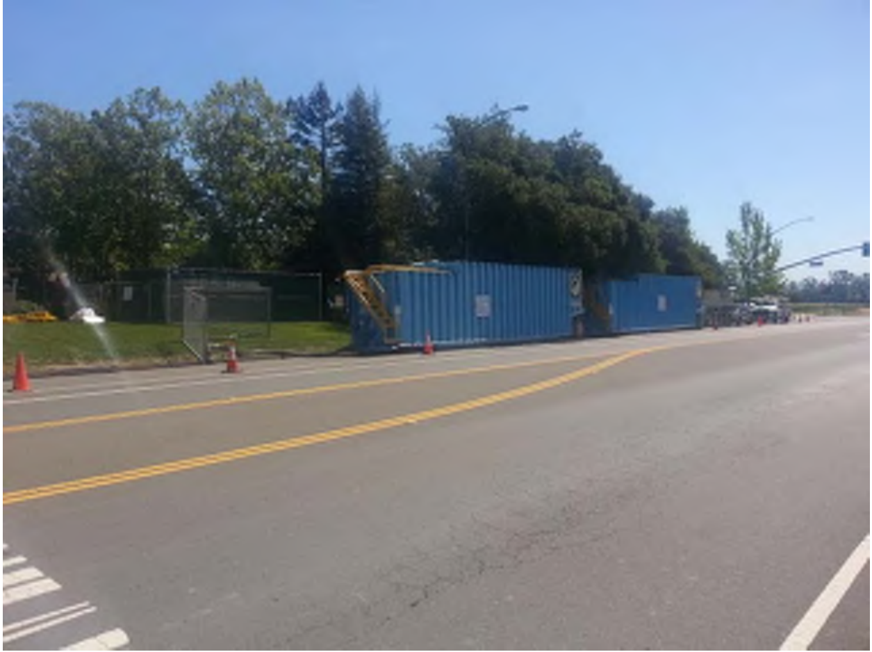
Baker tanks staged along Old Redwood Hwy used for settling of silt prior to filtration through bag filters.
